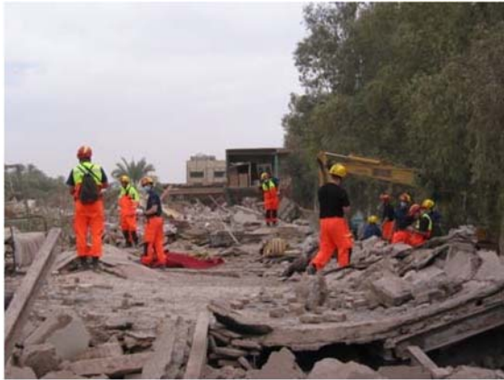
FRF performing a rescue at a collapsed building
